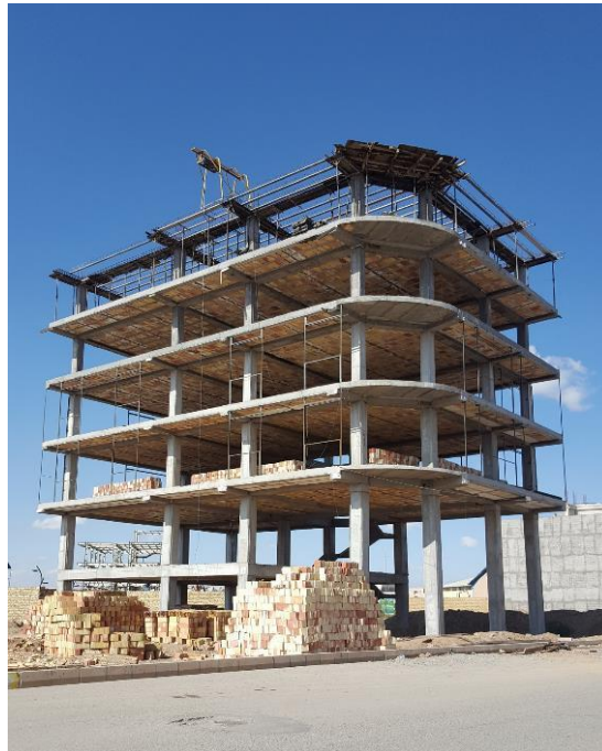
Figure 3 A residential structure with new materials and novel construction methods Source: Photo by Jahangirbakht, M.(2019). Takhti Street, Buin Zahra
