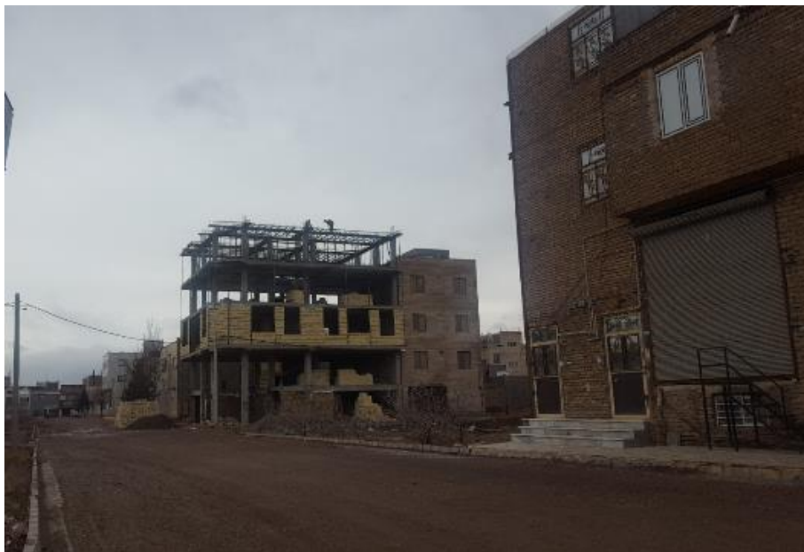
Figure 2. The structures being constructed of reinforced concrete along with the almost a complete and usable steel structure Source:Photo by Jahangirbakht, M.(2019). Farhang Street, Buin Zahra
