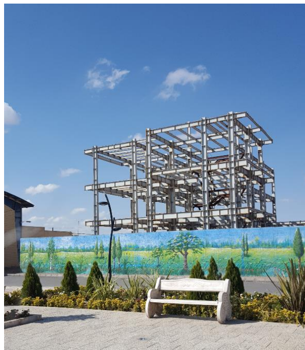
Figure 4. A structure with a bolted steel frame Source: Photo by Jahangirbakht, M.(2019). Takhti Street, Buin Zahra
