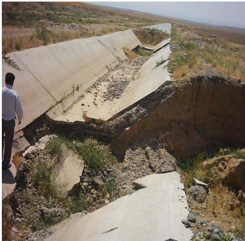
Figure 3: The destruction of pumping channel 3
